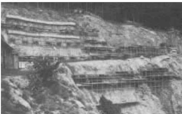
Fig. 12: Overall view of the slope during drilling operations in the middle section
