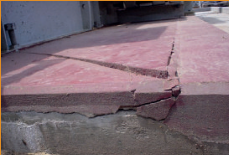
Grout cracking and edge lifting due to excessive grout placement, lack of expansion
